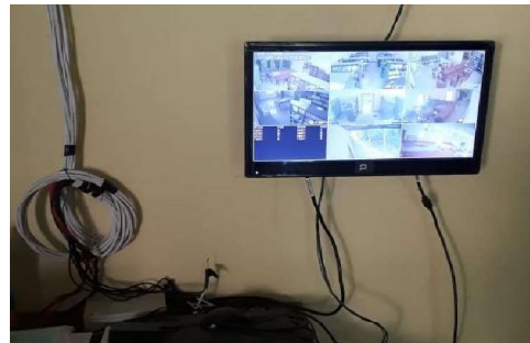
CCTV Surveillance at Library
